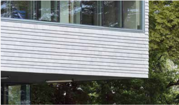
Koramic Plain Tile 301 White Glazed DLW architectes, FR - Nantes
