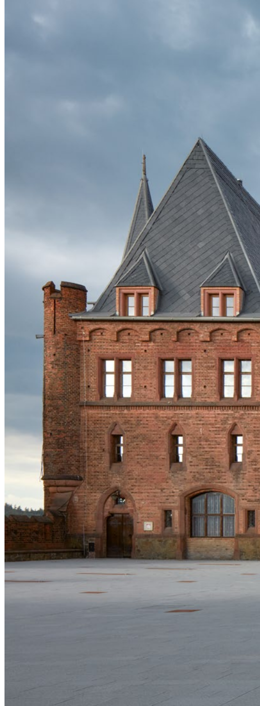
The first phase of reconstruction and monument-protection-compliant restoration concentrated on the structural renovation of the walls, vaults, lookout and roofs.
